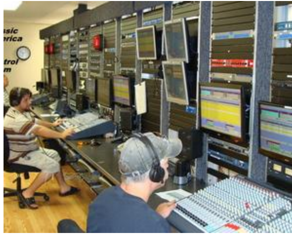
TOC, Technical Operations Center
